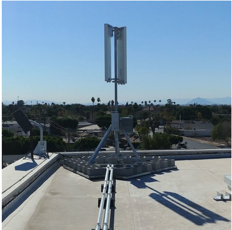
A “school-as-tower” installation at Brawley High School.
