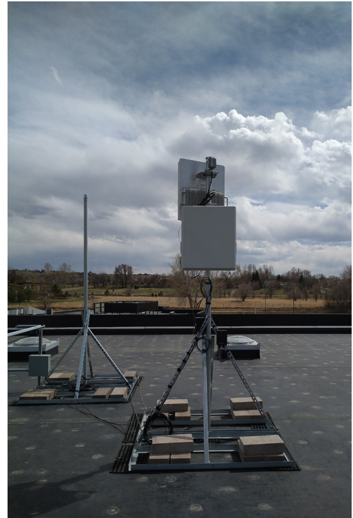
Cambium APs installed on a BVSD school rooftop Source: LiveWire
