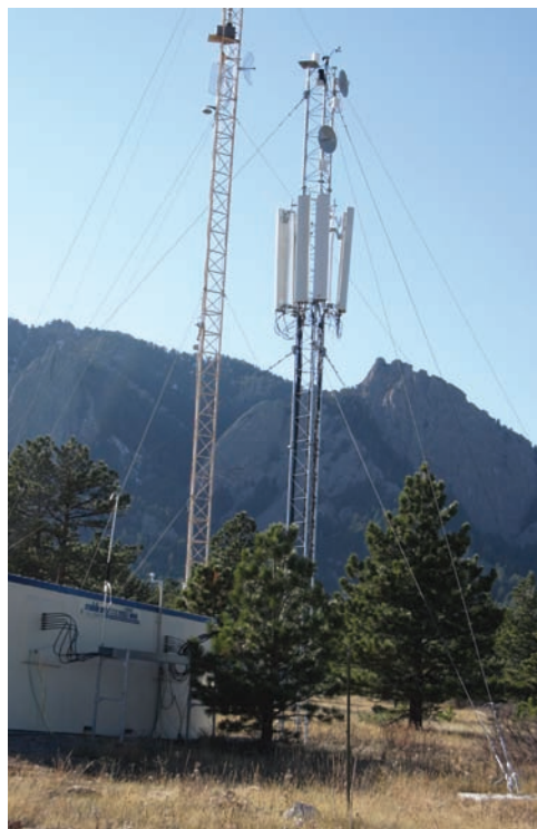
Antenna towers and control center at the Green Mountain Mesa Field Site. Photo by Ken Tilley.
