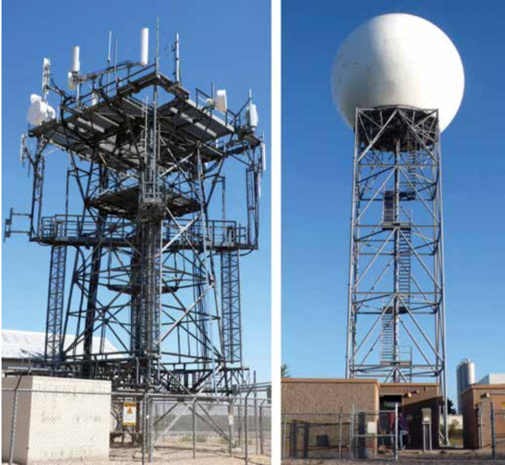
Left: A tower with communication transmitters that can interfere with NEXRAD weather radars. Right: A NEXRAD weather radar tower. Photos by Frank Sanders.
