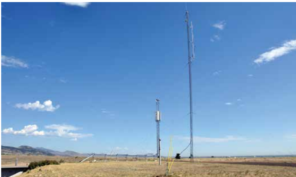
LTE antenna at the Table Mountain site—one of two fixed transmitters on the Public Safety 700 MHz Broadband Demonstration Network test network. Photo by Ken Tilley
