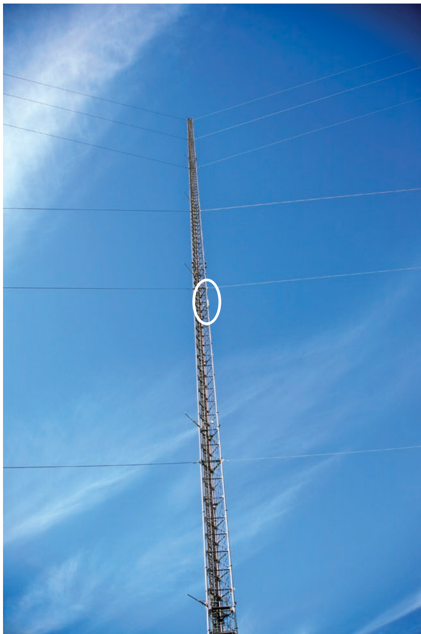
The 305 m “boomer” site mast. The test LTE base station antenna panel at 85 m above the ground is the white rectangle in the circle. Photo by Rob Stafford.
