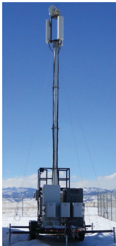
This cell-on-wheels (COW) is a component of the 700 MHz over-the-air (OTA) LTE network hosted and managed by ITS as part of the PSCR Public Safety Broadband test bed. Photo by Ken Tilley.
