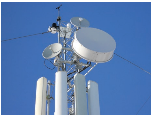
A cluster of antennas of various types used for testing of different telecommunications technologies at the Green Mountain Mesa Field Site. Photo by Ken Tilley
