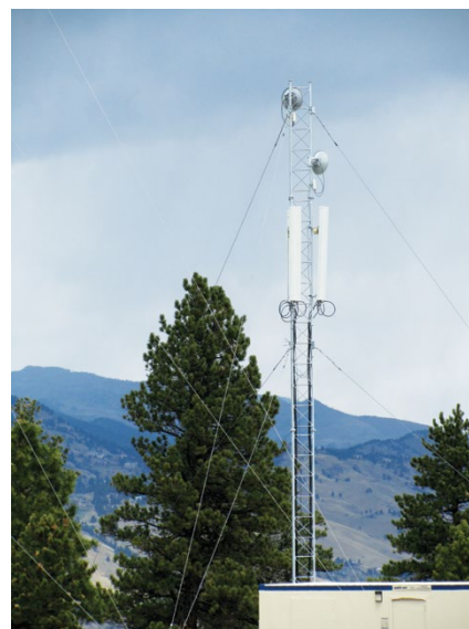
Antenna tower at the Green Mountain Mesa Field Site. Photo by Rob Stafford.
