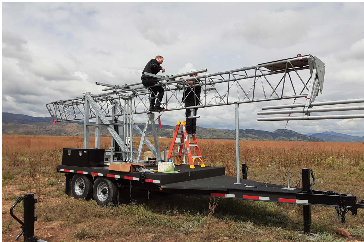
Specialized antenna face mount being installed by ITS's Kenneth Brewster (right) and Ryan McCullough on the mobile antenna tower at the Table Mountain mmWave 5G test cell site. (Photo credit: Jeffery Wepman).
