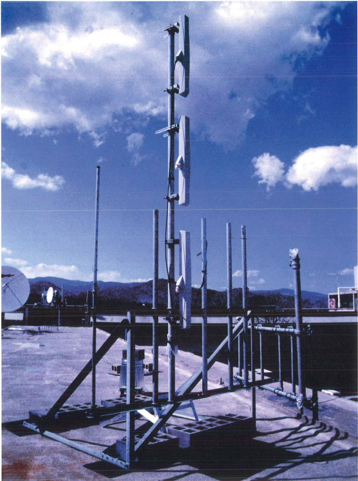
Vertical antenna array used by ITS adaptive antenna testbed (photograph by F.H. Sanders).
