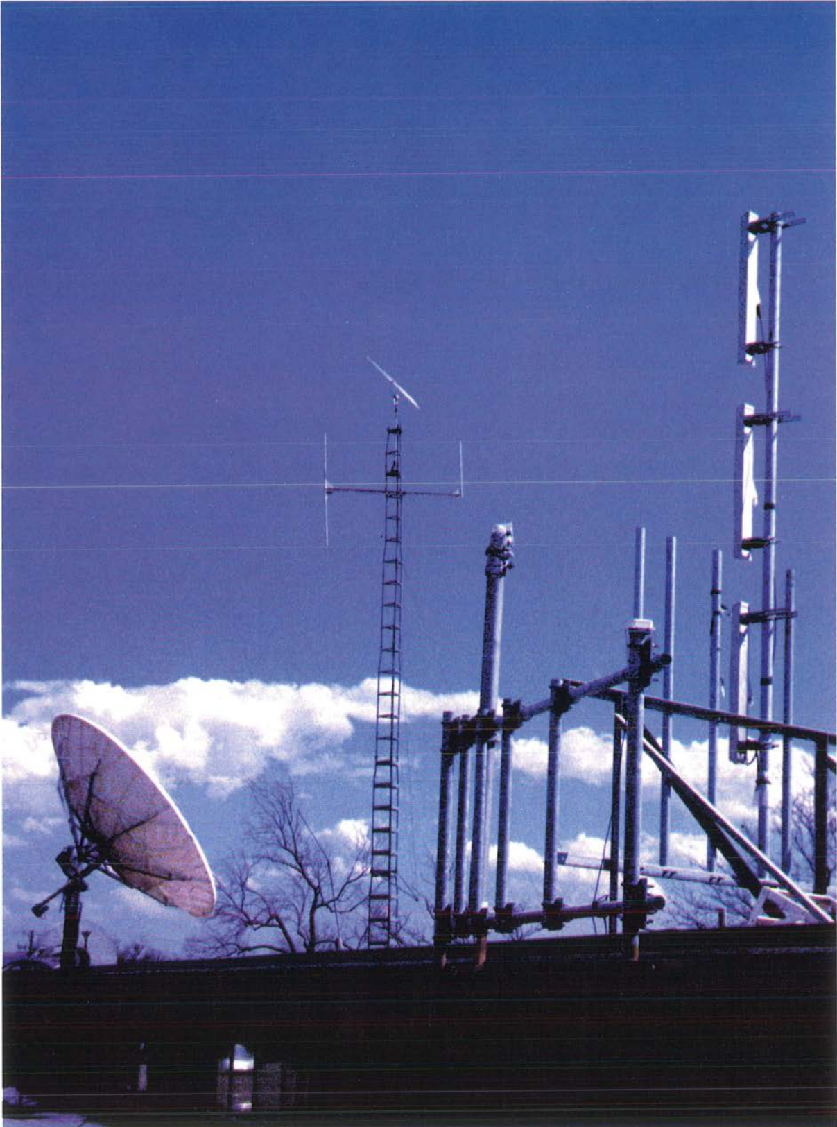
ITS antennas on the roof of the Department of Commerce Boulder Laboratories (photograph by F.H. Sanders).
