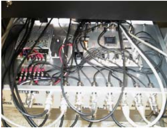
Figure 2. 16-channel FPGA P/N code generator at transmitter.
