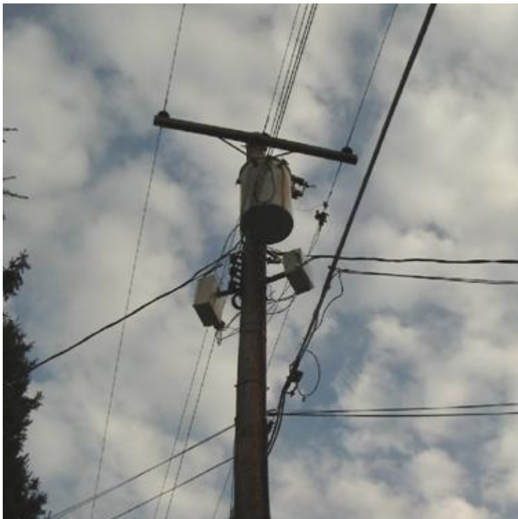
Figure 2-45: Multiple BPL devices located on the same utility pole
