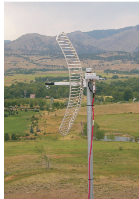
Figure 3. High gain directional antenna employed at one outdoor link at the Table Mountain field site (photograph by C. Redding).
