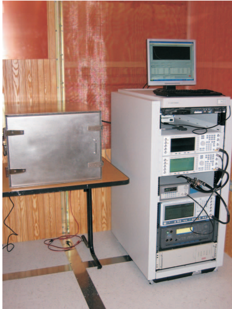
Equipment in the new ITS screen room (photograph by E. Nelson).
