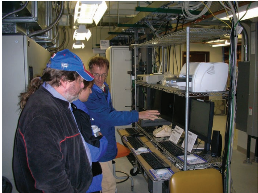
Figure 2. ITS personnel gathering LMR system information at an actual radio site (photograph by C. Redding).
