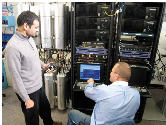
ITS staff examine the operational configuration characteristics of a Project 25 trunked LMR system in ITS' Public Safety RF lab.
