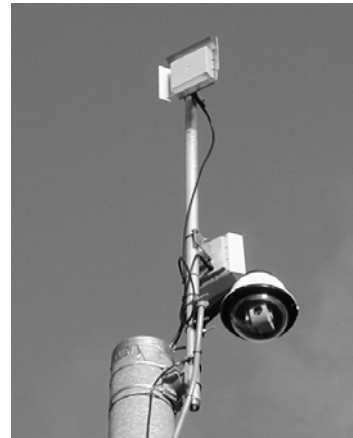
Figure 4 Typical installation of a repeater node and IP camera
