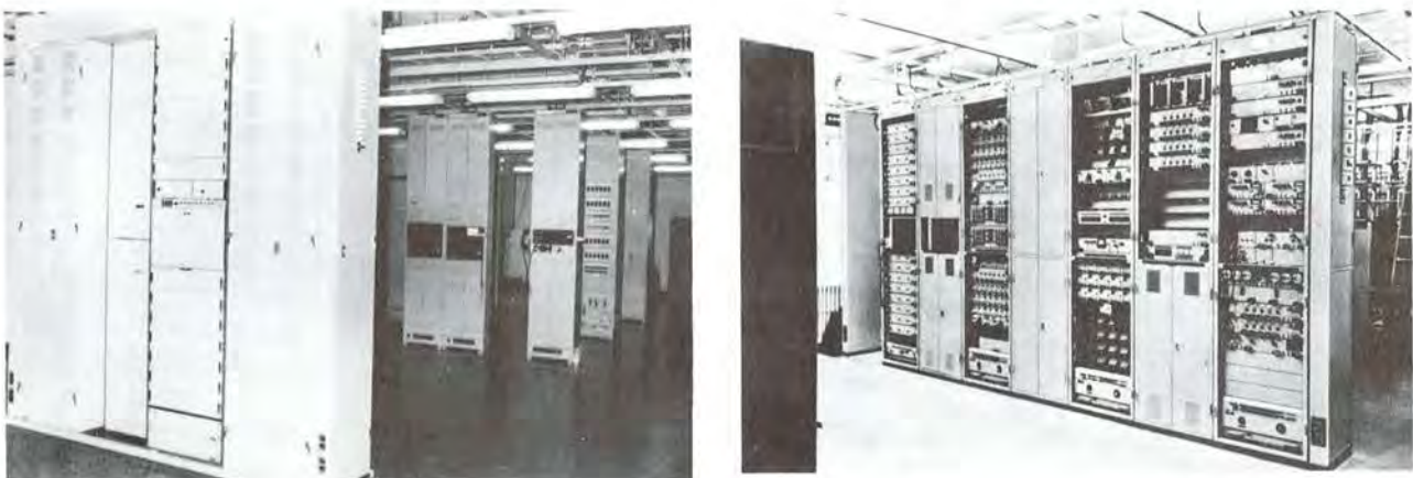
In appearance, submarine telephone cable system terminal station equipment resembles conventional telecommunication equipment enclosures, racks, cable-ways, and cabinets. With the surge in system channel capacity in recent years, the multitude of circuit terminations--per-circuit items-- would have been burdensome except for miniaturization stemming from solid-state technology, integrated circuit items, circuit-card techniques, etc.
