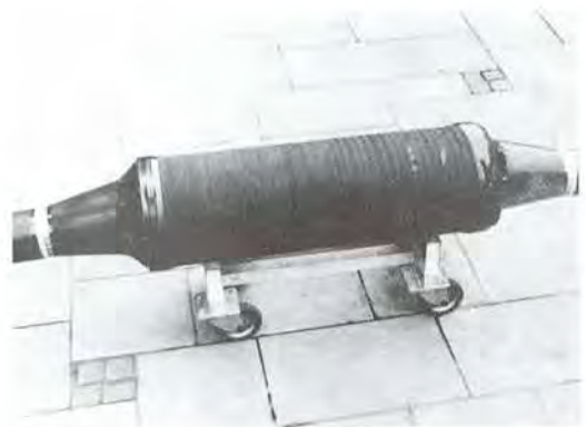
Repeater Ready for Enclosure in Shipping Container
